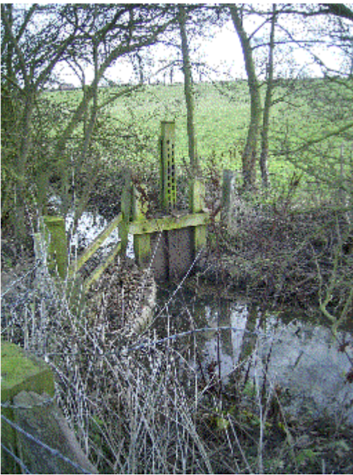
Picture, Sluice gate and feeder stream to control the supply of water to the canal.
